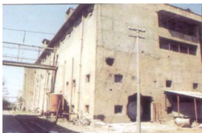
Photograph - A shows the building in which aluminium trays are installed. The building is specially designed with walls having abnormally high thickness (1000 mm) with height of about 15000 mm and a large built-up area.
