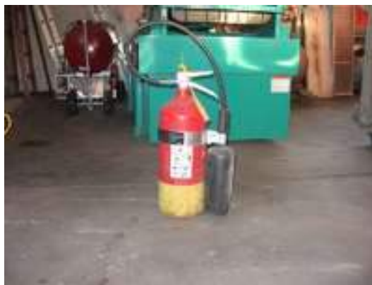
Carbon dioxide extinguisher
